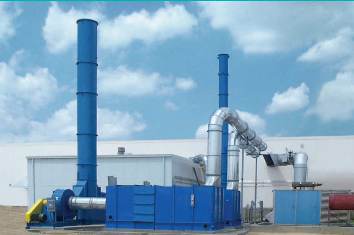
Mist Collectors, Dust Collectors and Scrubbers
